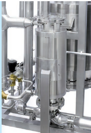
PSG 1500 T pre-heater using plant steam condensate
